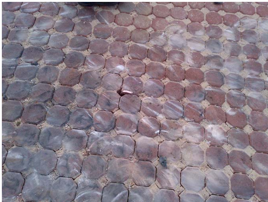
Figure 5. Close-up of tent spike location after being run over by the tank.
